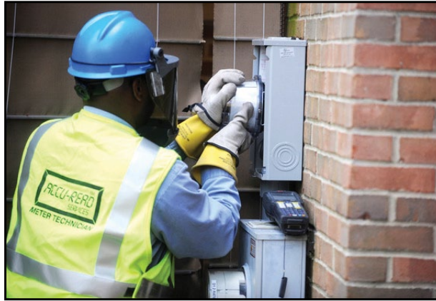
An Accu-Read Meter Technician installs a new DTE Energy smart meter at the home of an Ann Arbor resident.
